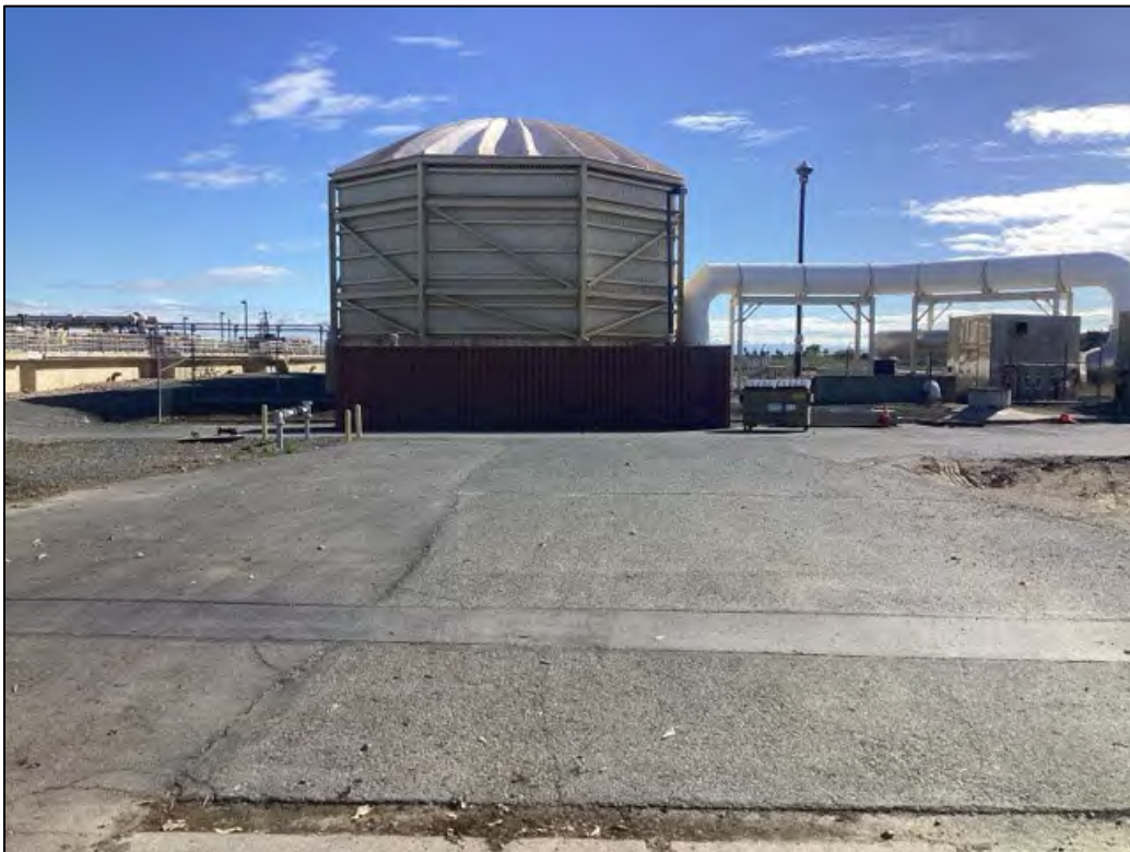
Photo 4. Aeration basin to be retrofitted (on far left) and trickling tower filters and odor control biofilter facility (center) to be demolished in project area within WWTP (looking east).
