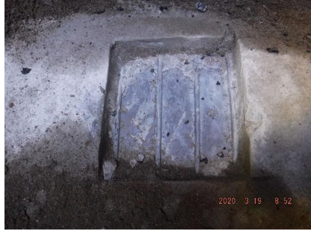
Photo 4-12. Exposed steel area at Location 5.
