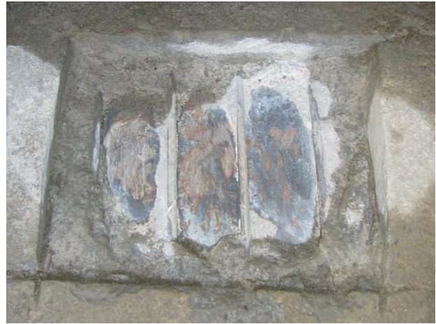
Photo 4-18. Exposed steel area at Location 13.
