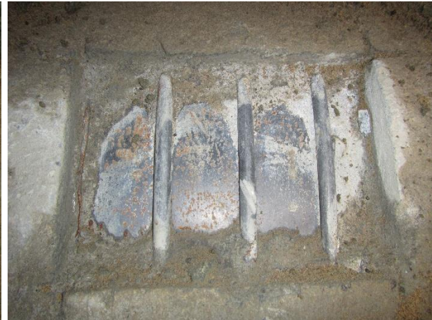
Photo 4-4. Exposed steel area at Location 9.
