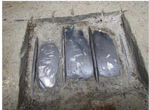
Photo 4-8. Exposed steel area at Location 2.
