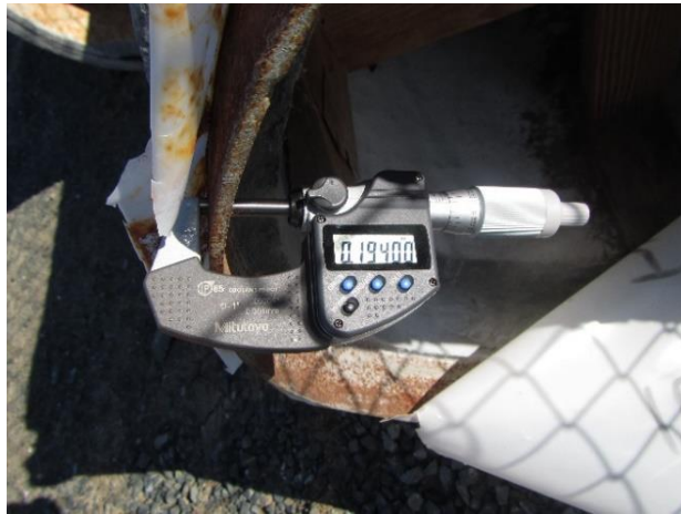
Photo 4-1. Replacement sections of pipe have a cylinder thickness of approximately 3/16 of an inch. The measured thickness was 0.194 inches, possibly including the rust.
