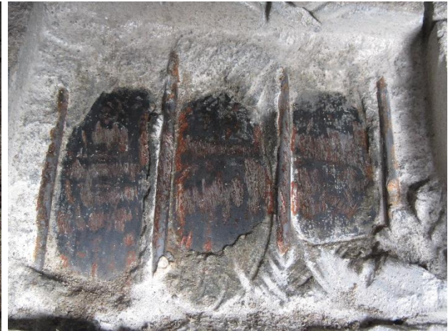
Photo 4-6. Exposed steel area at Location 1.
