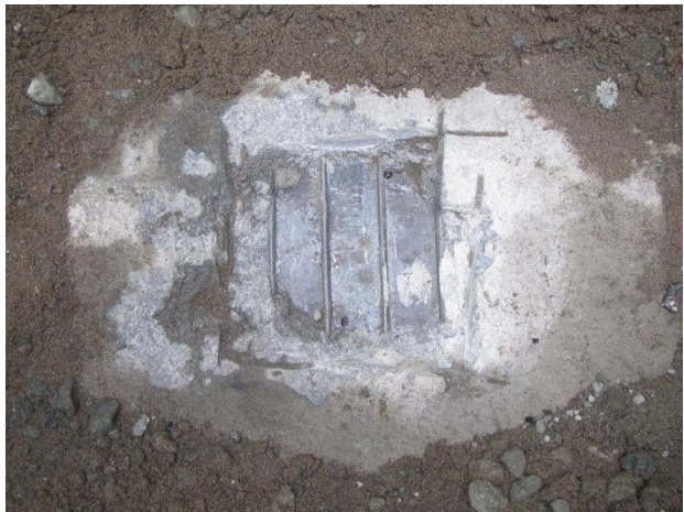
Photo 4-19. Exposed pipe surface at Location 14, as found. North is to bottom of photo.
