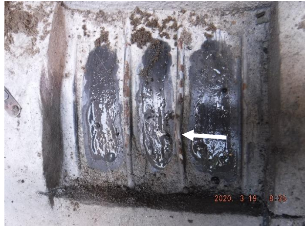
Photo 4-14. Exposed steel area at Location 6. Surface is wet from ultrasonic testing. Note bent bar (arrow).
