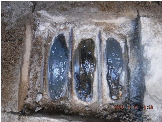
Photo 3-1. Typical area of steel cylinder exposed at the crown of the pipes for ultrasonic thickness testing. The wet surface is the couplant used to ensure that the ultrasonic waves pass into the metal.
