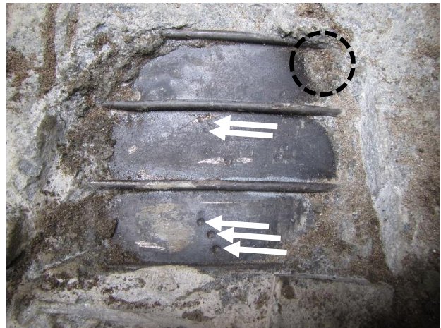
Photo 4-20. Exposed steel area at Location 14. Dimples denoted with arrows. Dent (as found) circled with dashed line. North is to left.
