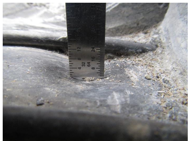
Photo 4-22. Dent at Location 14 is about 3/16 to 1/4 of an inch deep.
