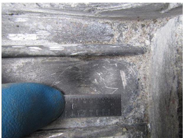
Photo 4-21. Dent at Location 14 is about 1 inch in diameter.
